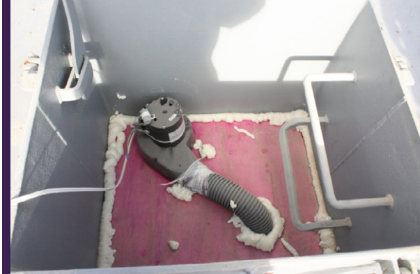
Recirculation fan positioned in hold access trunking
